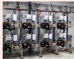
Example of an installation.
